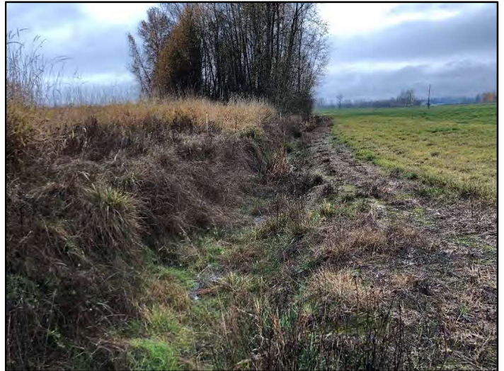
Photograph 6: Standing water observed in drainage ditch at the west parcel boundary of parcel no. 214247000, running north-south.
