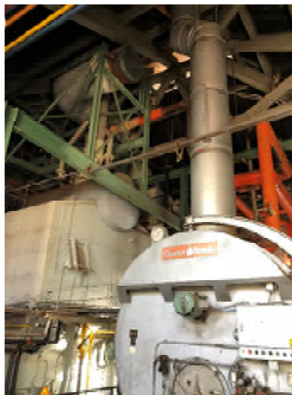
Boiler House equipment and interior structural frame
