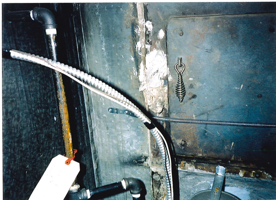
B. ASBESTOS-CONTAINING CEMENT MATERIAL; BASEMENT FURNACE UNIT.
