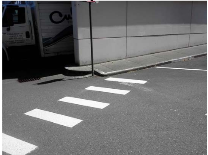
Photo 8. No Curb Ramp
