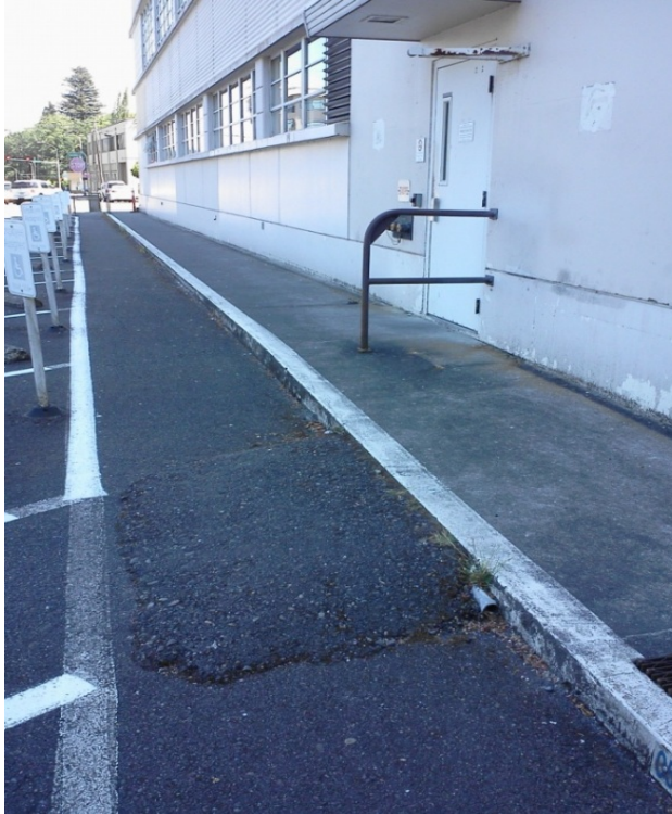
Photos 3. Railing Encroachment
