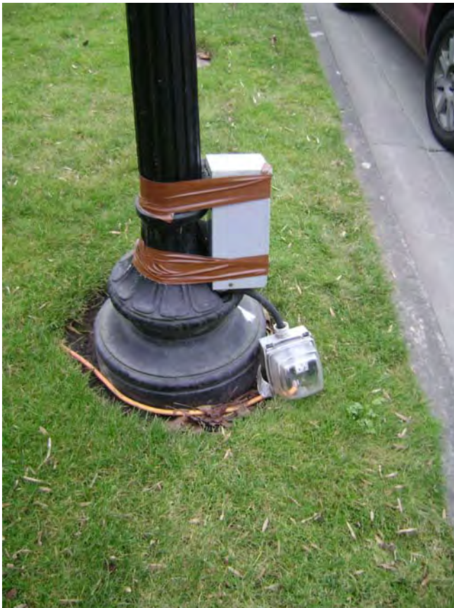
Figure 11.3 Electrical outlet attached to light pole base as observed during site survey (source: Dark|Light Consulting, LLC, 2009)
