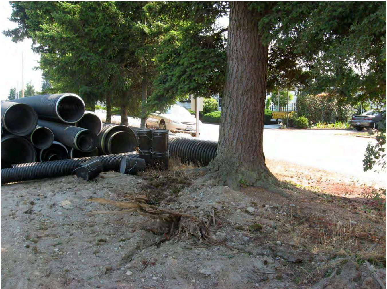
Fig. 10.6.1 Careful drainage system planting & installation could have prevented tree root damage. (August 2005, Source: Arbutus Design)
