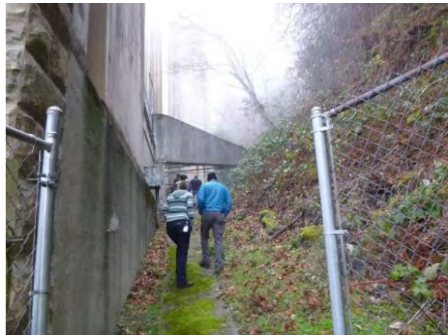
Figure 1. Steep Slope Adjacent to Central Plant
