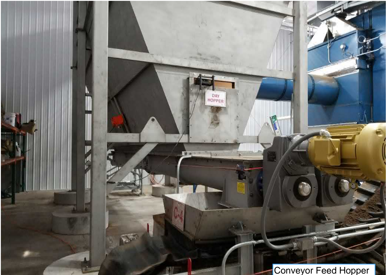
Conveyor Feed to Thermal Unit
