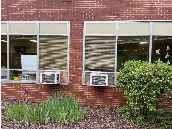
Package air conditioners retrofitted into the existing windows
