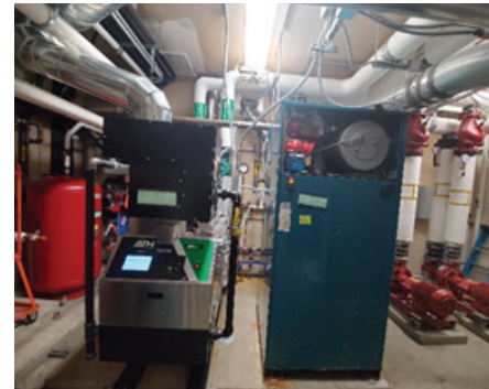
The (2) new 1,600 MBH boilers on see on the right. Existing heating water pumps and boiler flues were retained. New assembly is under warranty to the same manufacturer and to the same installer.
