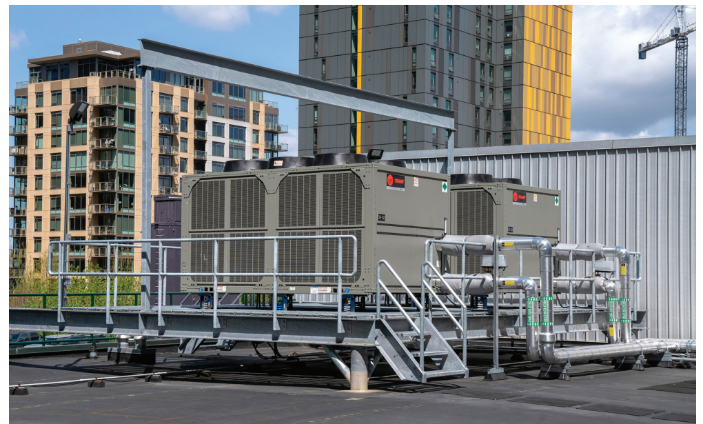
New platform and chillers
