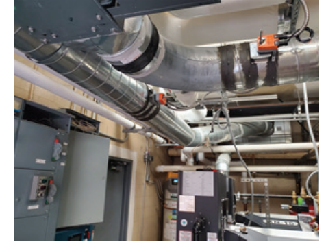
The 1,600 MBH boiler on the left was installed under an Emergency Project. The new boiler was linked to the existing 3,000 on the right so the College would retain heating water redundancy.
