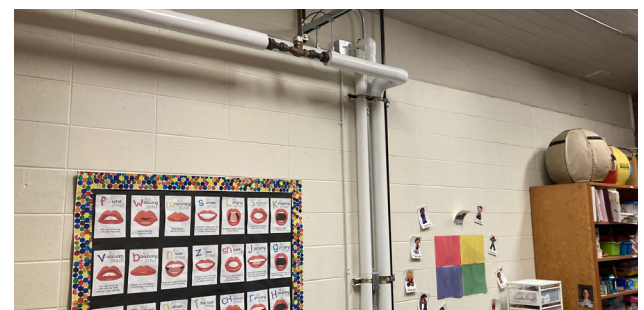
SEATTLE PUBLIC SCHOOLS NORTH BEACH ES | HVAC & FIRE SPRINKLERS
