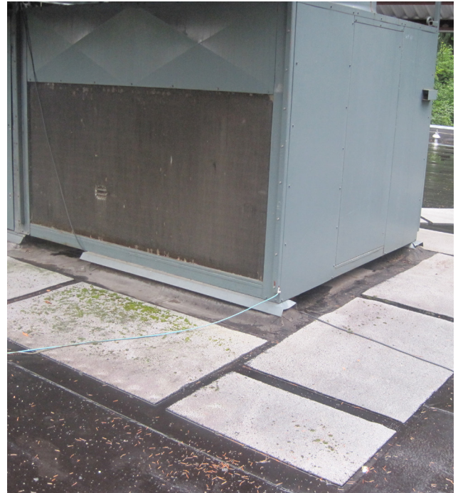
GREEN RIVER COLLEGE AD BUILDING | ROOFTOP HVAC UNIT
