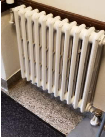
Cast Iron Radiator
