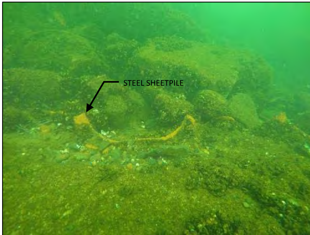
Photograph 14: Rock Armoring at North Edge of Spillway, Cut Off Steel Sheetpile in Foreground
