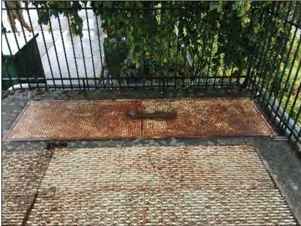
Photograph 30: Condition of the Stillwell Hatch Cover
