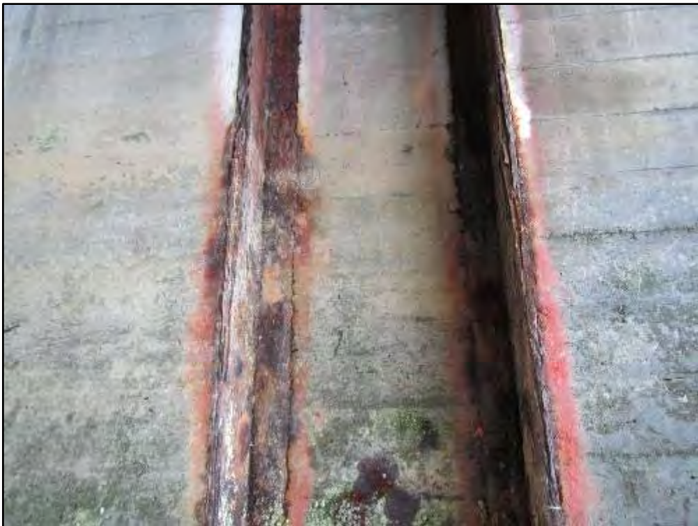
Photograph 11: Stoplog Cutout with Moderate Corrosion
