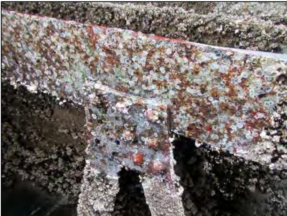
Photograph 21: Minor Corrosion on Radial Gate in Intertidal Zone
