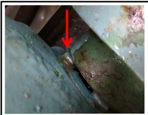
Figure 2-11 Coupler Proximity to Gearbox –West Gate
