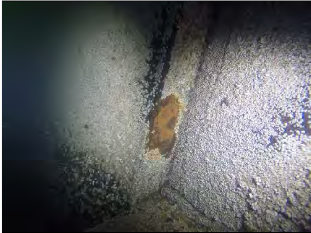
Photograph 48: Moderate Corrosion on Stoplog Cutout on Downstream Side
