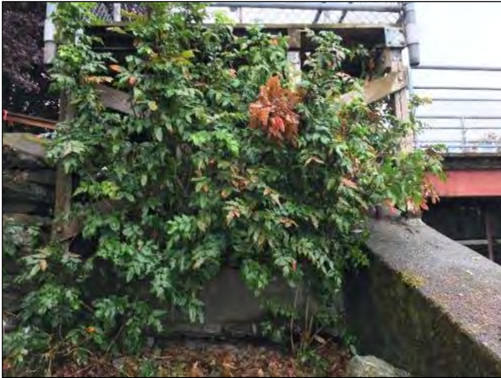
Photograph 27: The Concrete Retaining Wall Supporting the Walkway Exhibits Moderate Undermining
