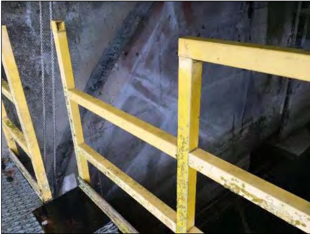
Photograph 52: Missing Catwalk Guardrail Top Rail on the West Side of the West Spillway
