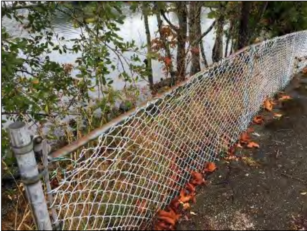
Photograph 50: Disconnected Top Rail at the West end of the Concrete Ramp
