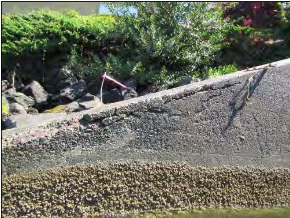
Photograph 6: Open Corrosion Spall on East Downstream Wingwall
