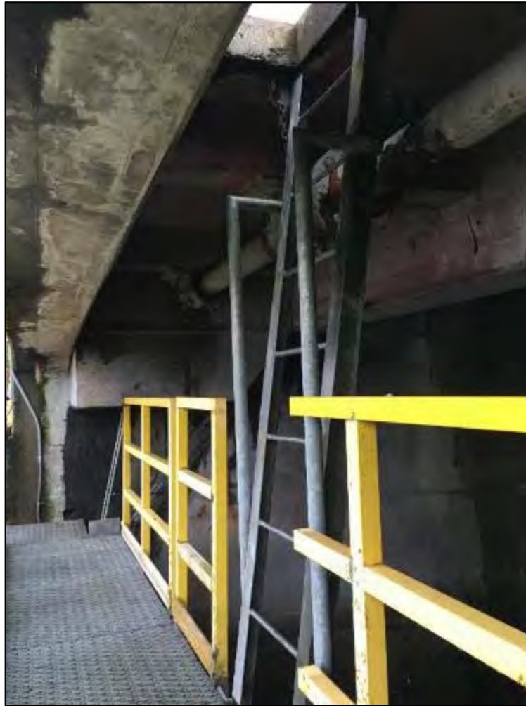
Photograph 32: Condition of the Catwalk Access Ladder
