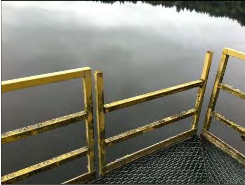
Photograph 35: Missing Top Rail Near the Center of the Catwalk
