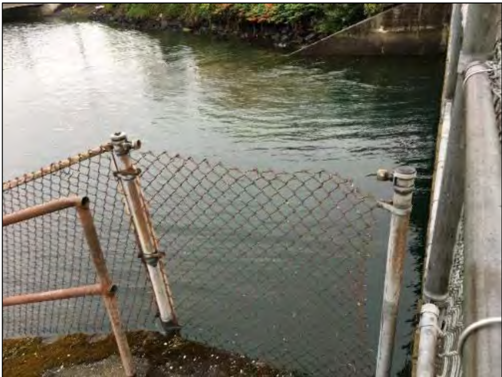
Photograph 49: Missing Top Rail on the Northwest Wingwall Fence
