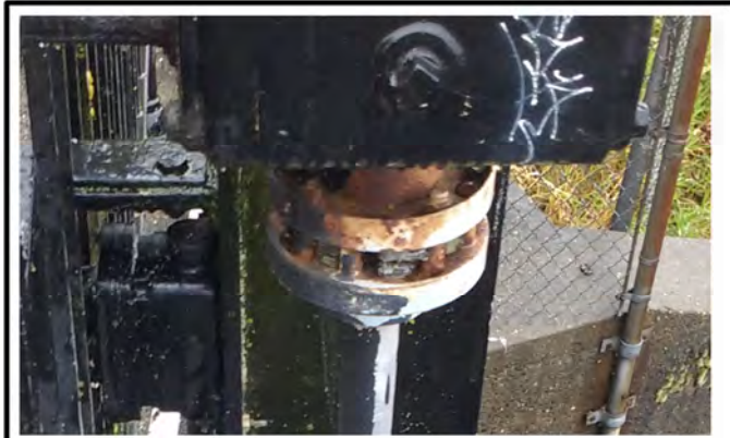
Figure 2-27 Exposed Coupling with Degraded Elastomer
