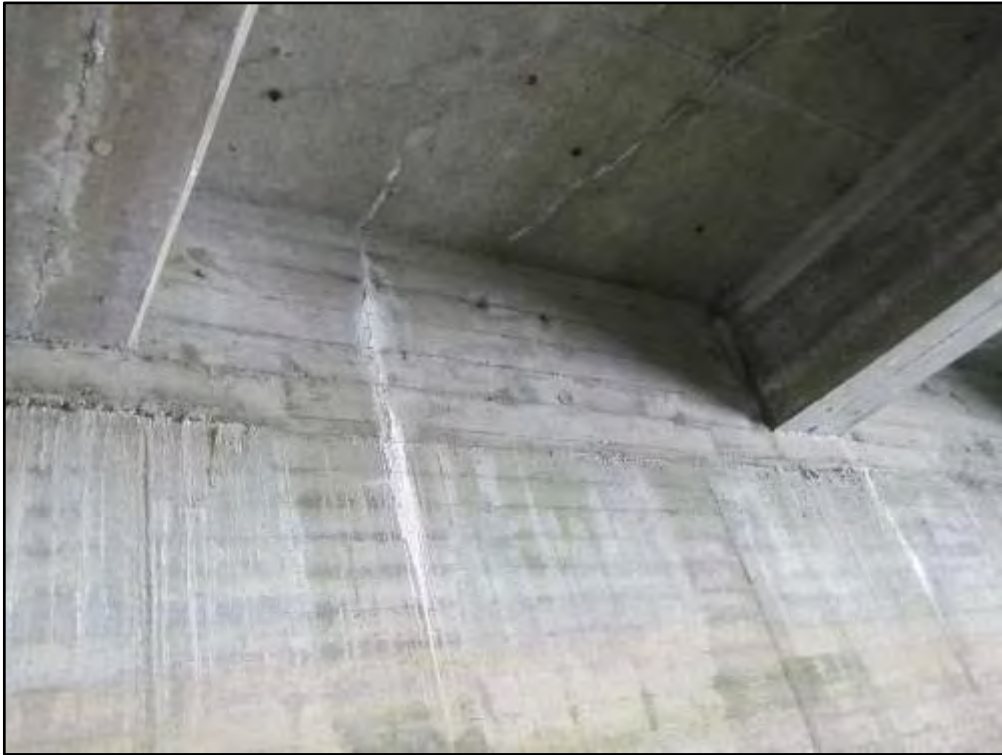
Photograph 5: Efflorescence on West Abutment
