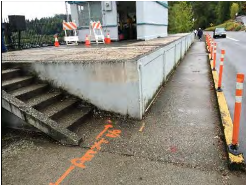
Photograph 37: No Handrail Along the Edge of the Elevated Platform and Steps
