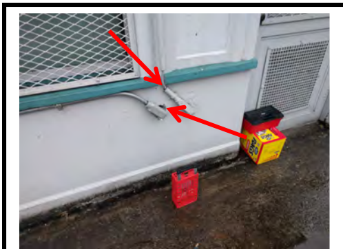
Figure 2-32 Water ingress via conduits
