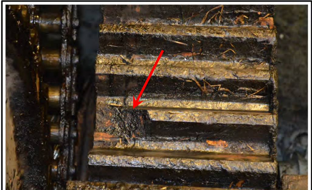
Figure 2-6 Broken Tooth – Pinion Gear – East Tide Gate
