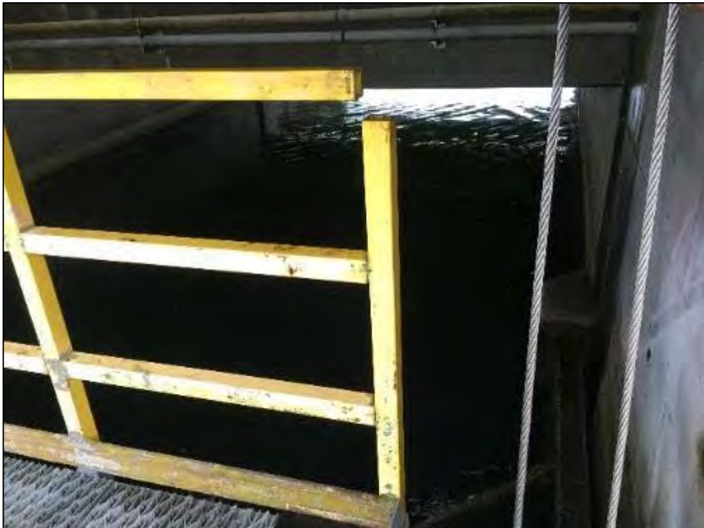
Photograph 51: Missing Catwalk Guardrail Elbow on the East Side of the West Spillway
