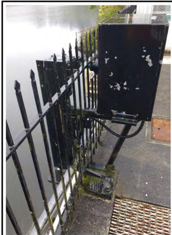
Figure 2-26 Gearbox Enclosure and Switch
