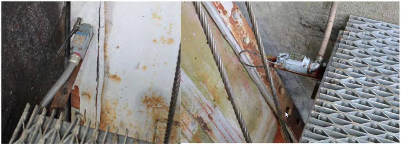
Figure 2-5 Back-up Limit Switches – Tide Gates
