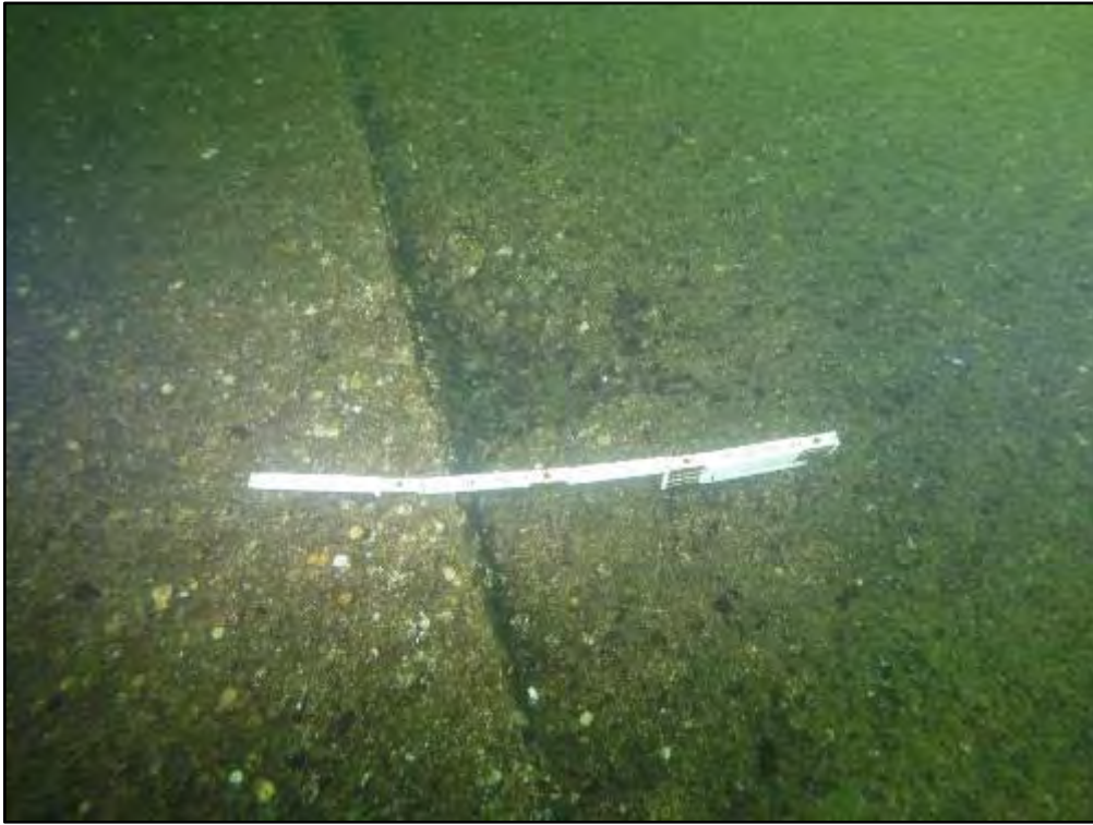
Photograph 10: Spall on Bottom Slab at Expansion Joint
