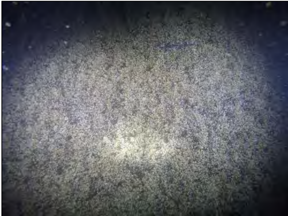
Photograph 9: Typical Marine Growth on Concrete Surfaces Underwater
