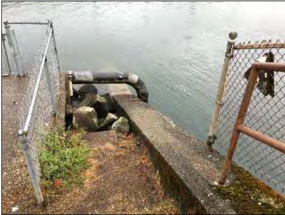
Photograph 38: No Fence Between Concrete Ramp and Wingwall Fence
