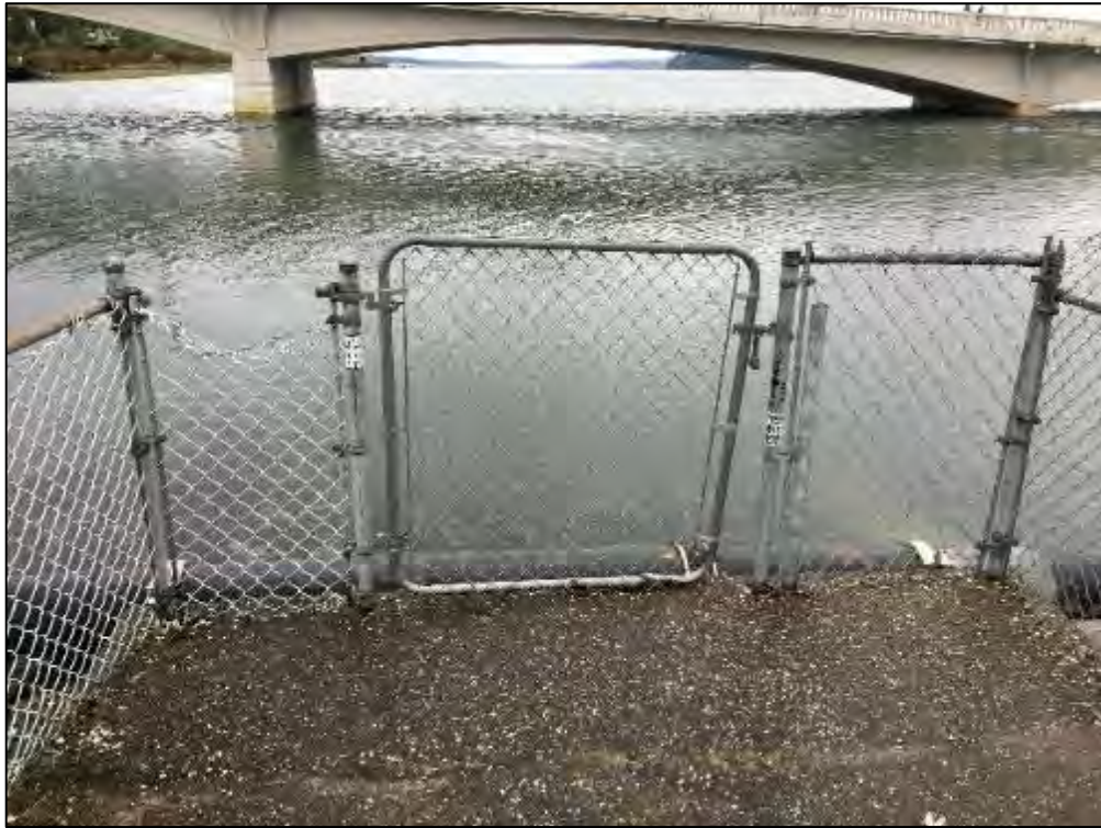
Photograph 36: Missing Top Rail on the Concrete Ramp
