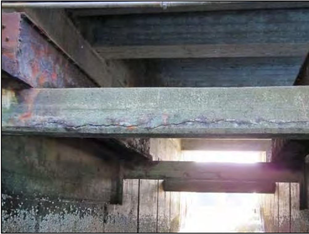
Photograph 17: Typical Closed Corrosion Spall on Fish Channel Crossbeam
