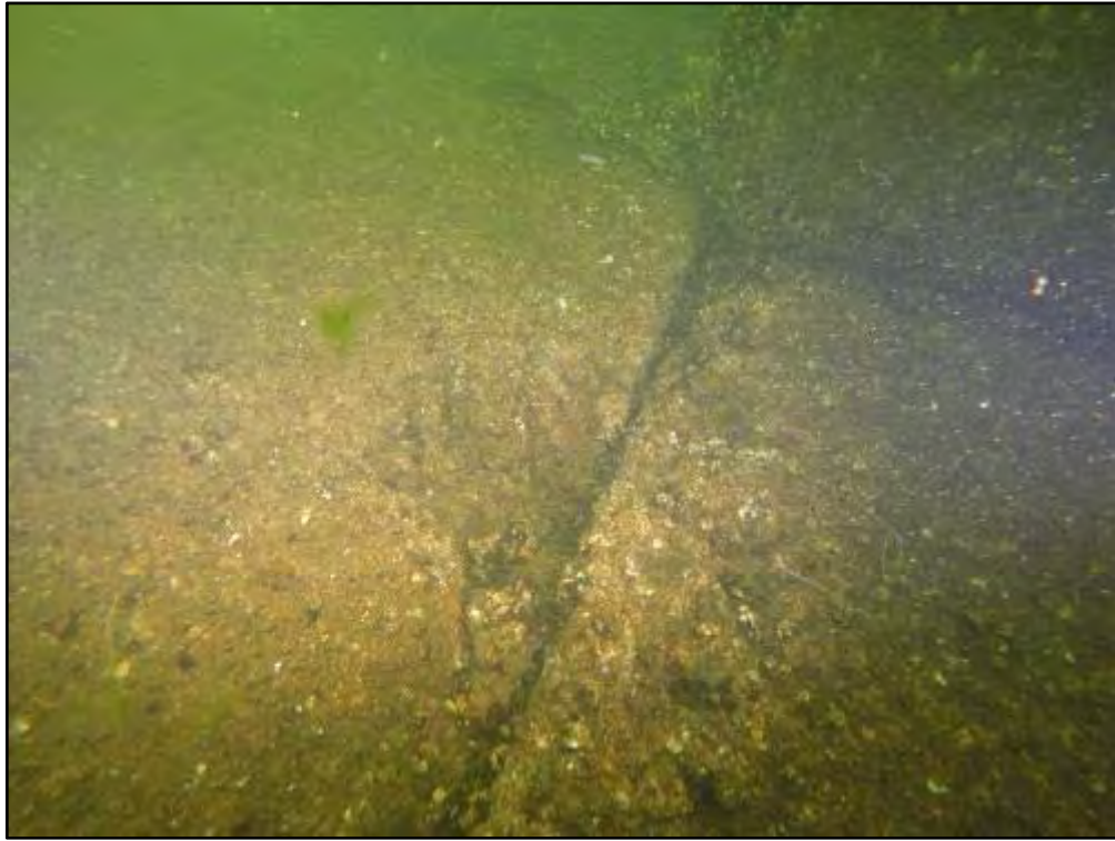
Photograph 46: Spall on Bottom Slab at Expansion Joint
