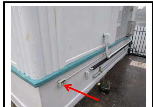
Figure 2-33 Electrical Shock Hazard, Energized Parts Exposed to Public
