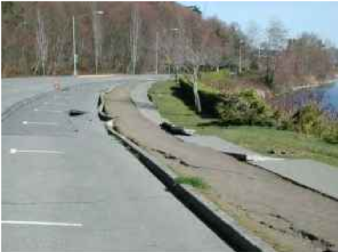
LIQUEFACTION-RELATED DAMAGE FROM (a) THE 1965 SEATTLE-TACOMA EARTHQUAKE (b) THE 2001 NISQUALLY EARTHQUAKE (KRAMER 2008). NOTE THAT BOTH PHOTOGRAPHS WERE TAKEN AT ABOUT THE SAME LOCATION ALONG DESCHUTES PARKWAY SW.
