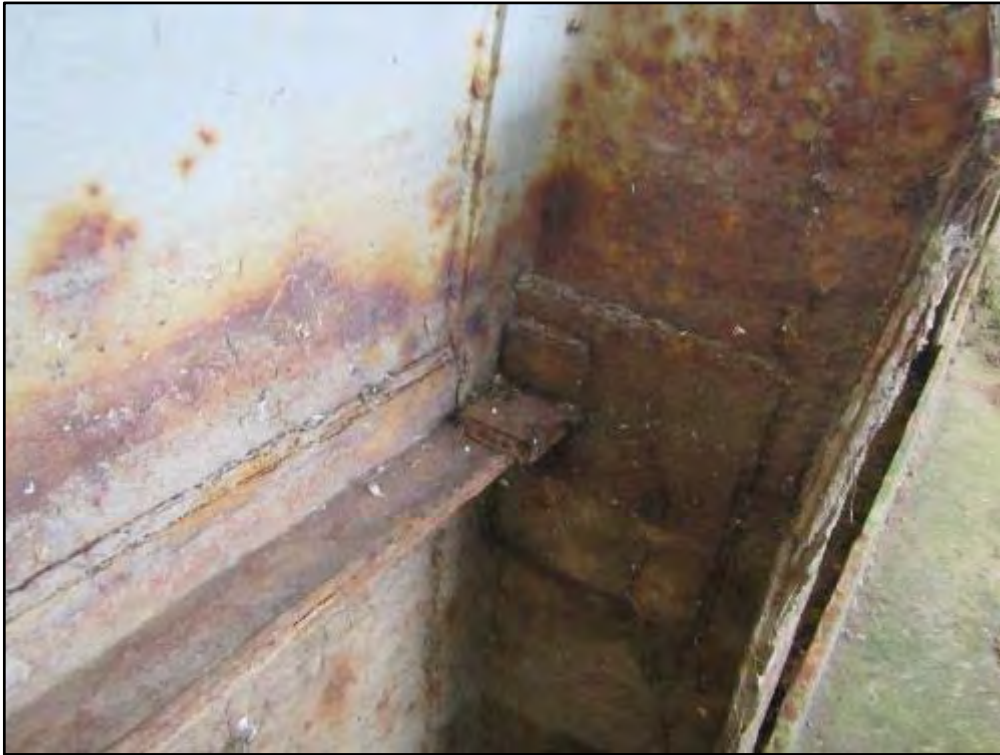
Photograph 20: Moderate Corrosion on Radial Gate Above Water
