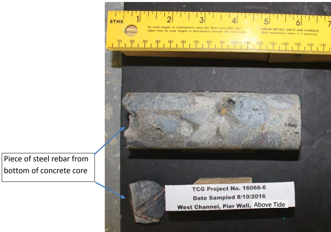
Figure 30: Sample 6 – Pier Wall Above Tide
