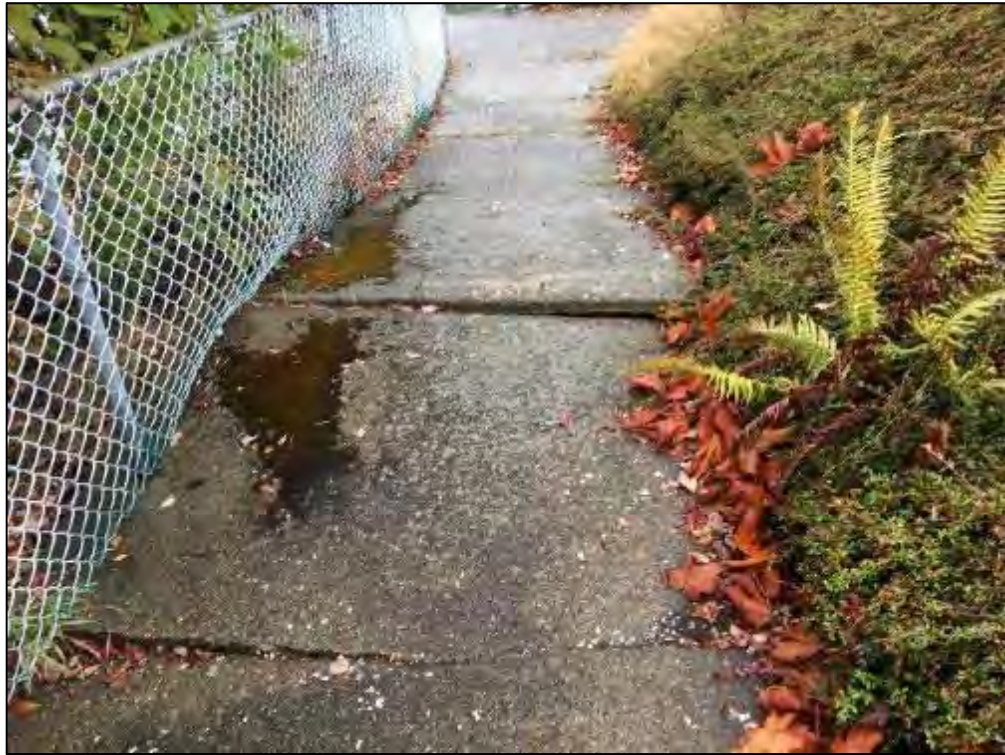
Photograph 28: The Concrete Ramp Exhibits a Large Bump Extending Approximately 10 Feet and has a Vertical Differential of Approximately 12 Inches.
