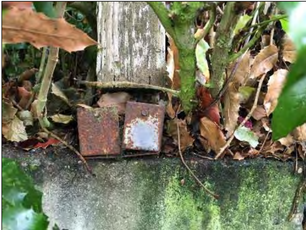
Photograph 26: Timber Post Exhibits Rot and Section Loss and the Steel Connection is Corroded and Deformed
