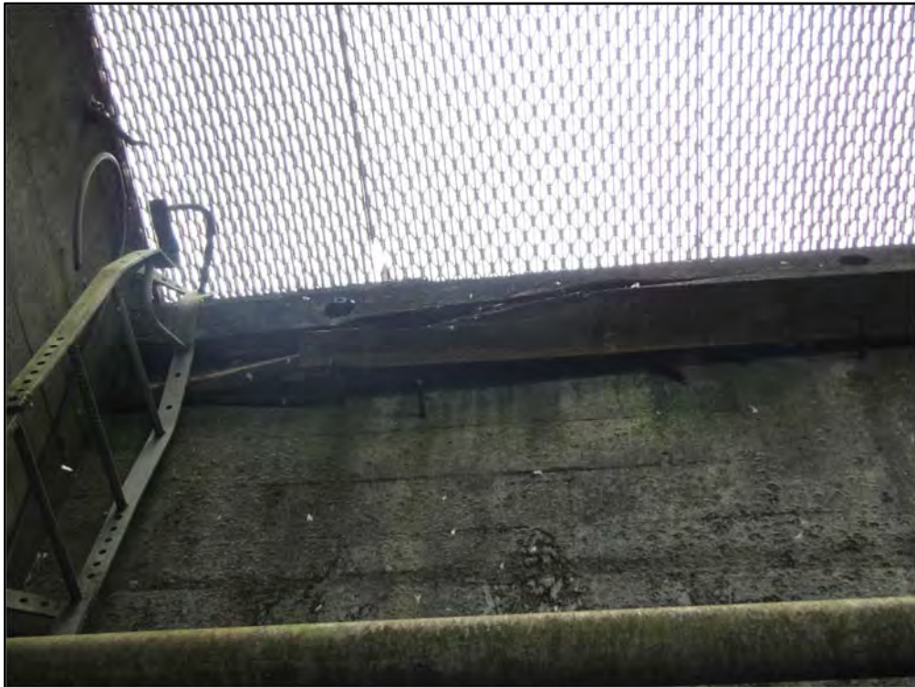
Photograph 34: Crushed Timber Cushion and Deformed Radial Gate Access Ladder
