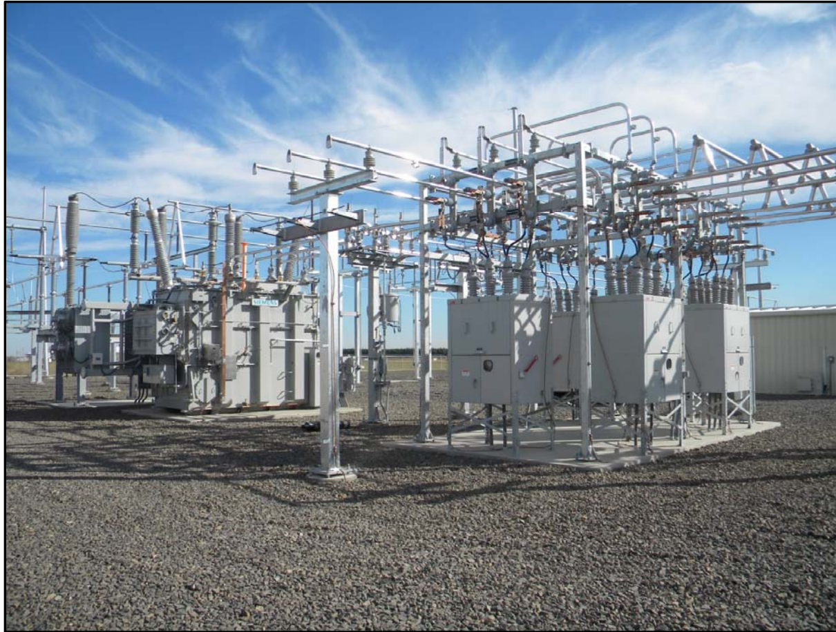
Substation Reliability Project, Cloud View Substation, Completed 2017
