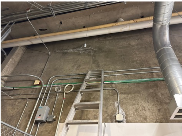
Detail of interior leak caused by the cracks at the exterior basin.
