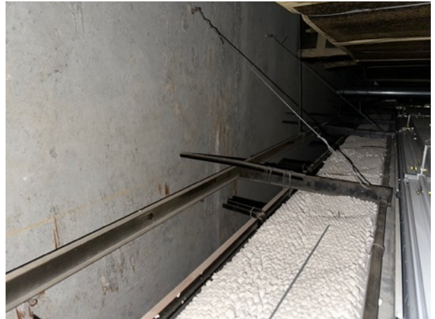
Detail of the top of the wall showing plaster and lath construction with metal tie supports.
