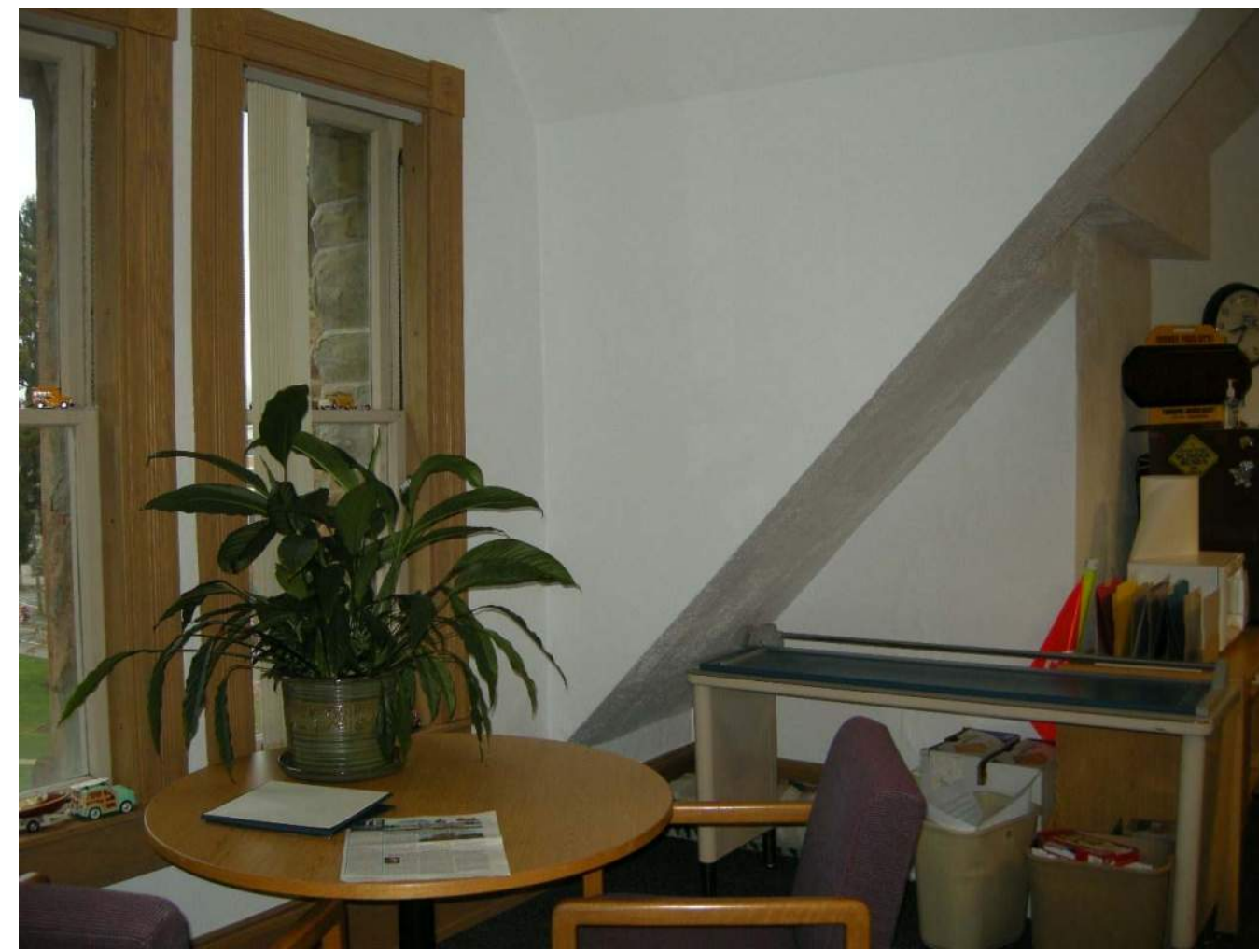
7 (e) Condition - Damaged Plaster at Dormer
