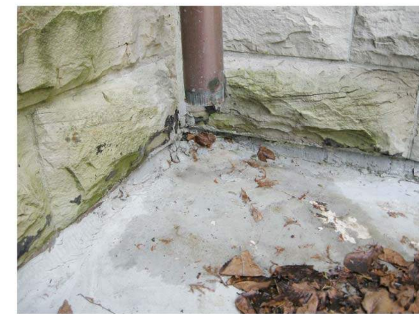
9 (e) Drainpipe at Northwest Corner of Mech. Room Existing Conditions
