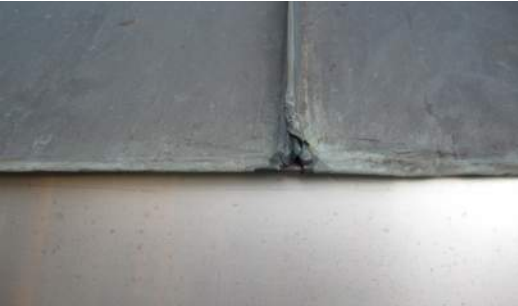
Figure 3. Torn pan at roof eave
