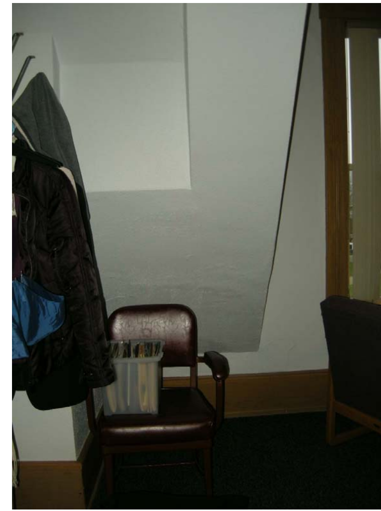
4 (e) Condition - Damaged Plaster at Dormer
