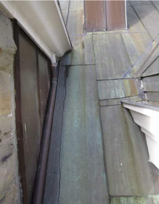
Figure 2. Water leaking at pan hem
