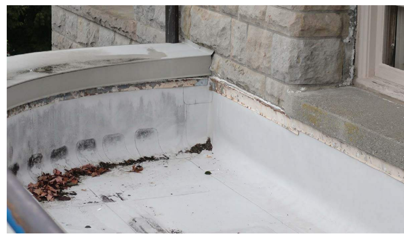
1 Balcony Flashing Existing Conditions
