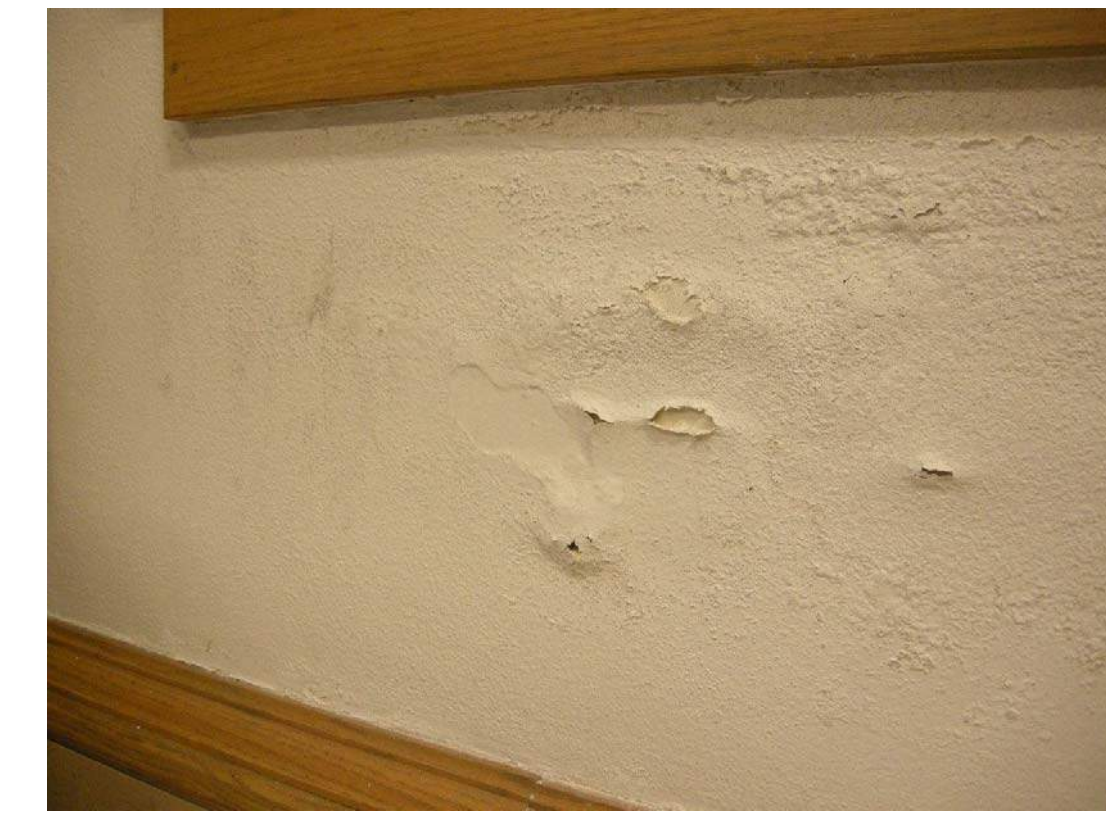
15 (e) Condition - Damaged Plaster
