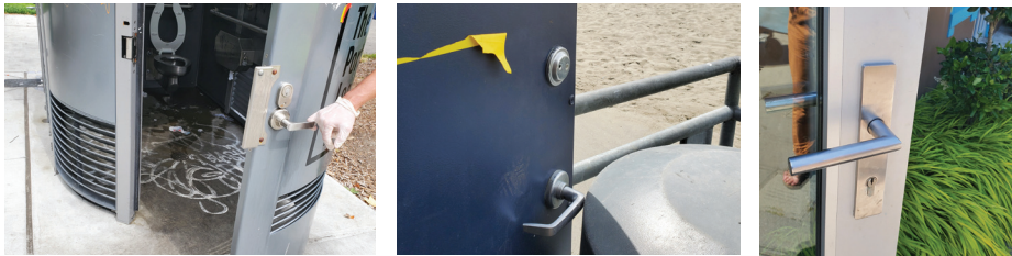
Left: Vandalized hardware; Middle: Lockset damage by Sand; Right: Failed Hardware at SCPG
