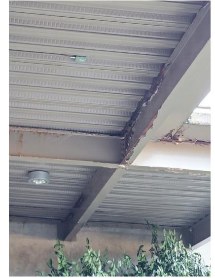
Left: Repaired 9000 Building; Right: Water damage soffit
