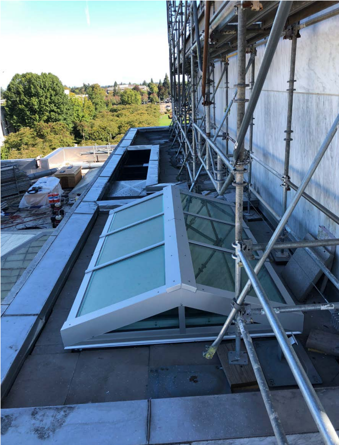
View of the new skylight over historic concrete and wired glass skylight
