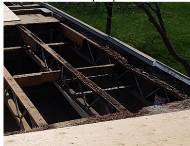
Decayed roof joist (requiring replacement)
