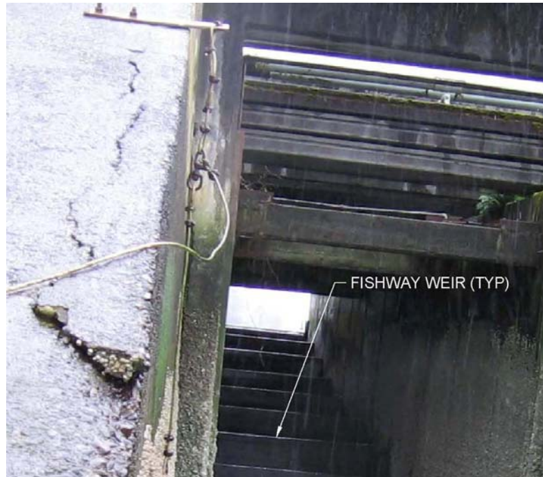
Figure 7. Spalled Downstream Wing Wall
